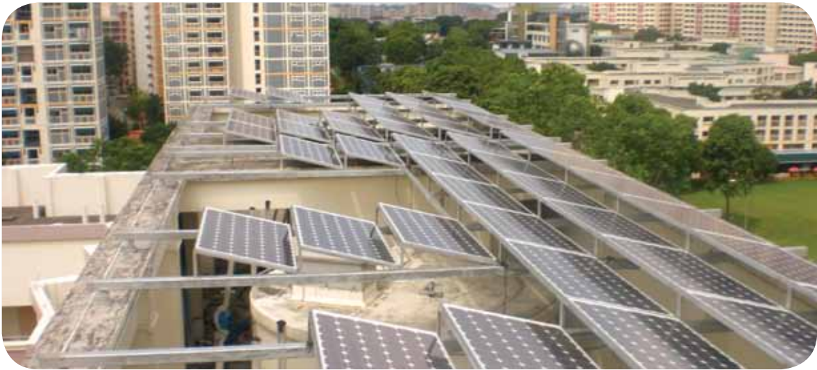
Fig. 4.1 Solar PV system on a HDB building
