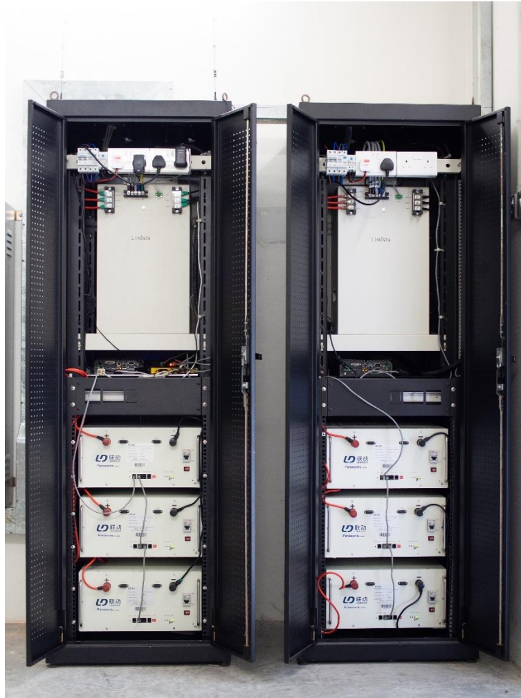
Distributed ESS deployed within a switchroom in Punggol
