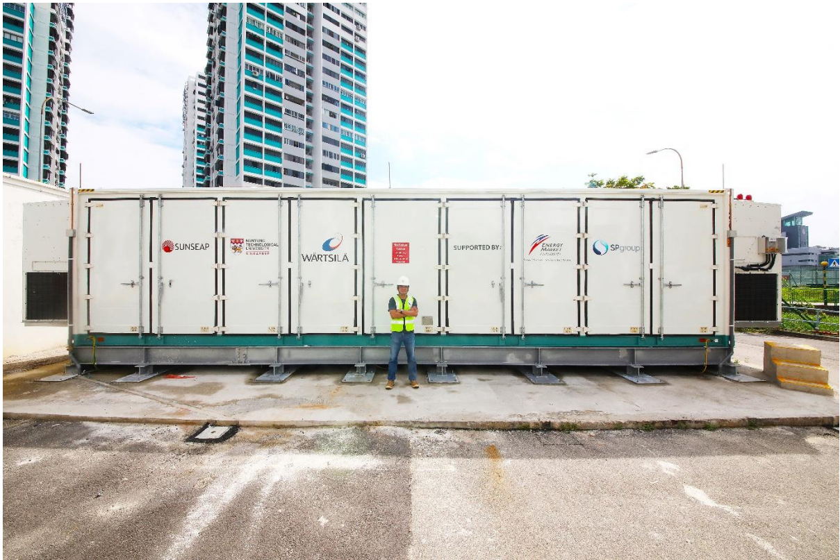
Photos of Singapore's first Utility-Scale Test-bed
