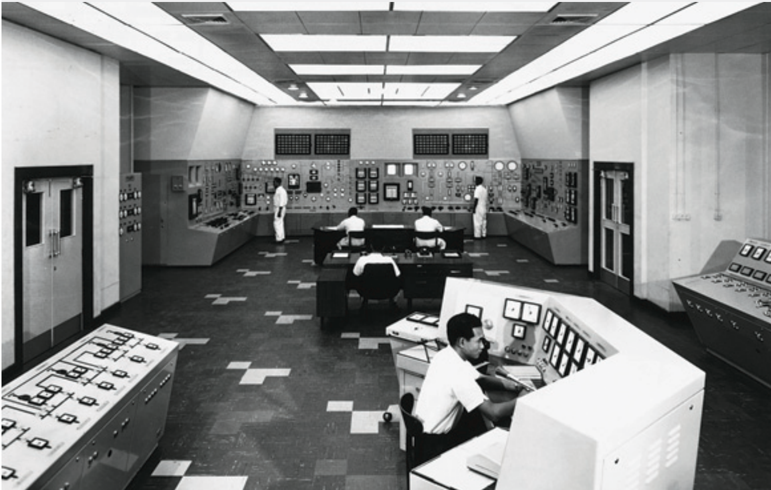
An electricity distribution centre monitoring demand spike.
